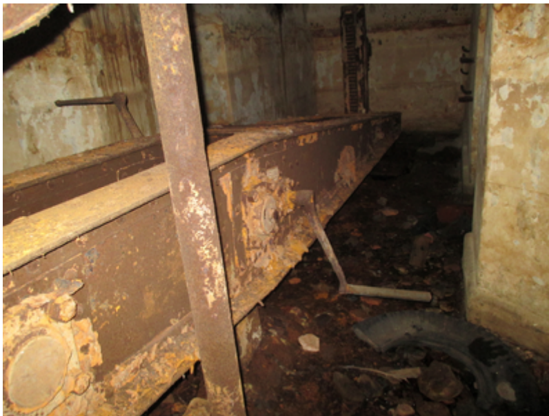
The reverse of the previous, looking back toward the jack. Showing the pivot point and the jacking arms.
