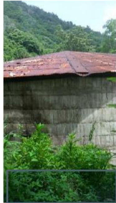
Side view of the tank
