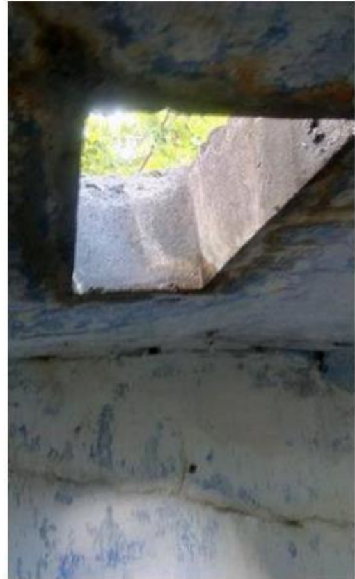
Looking up at the air vents
