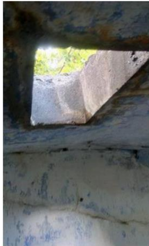
Looking up at the air vents
